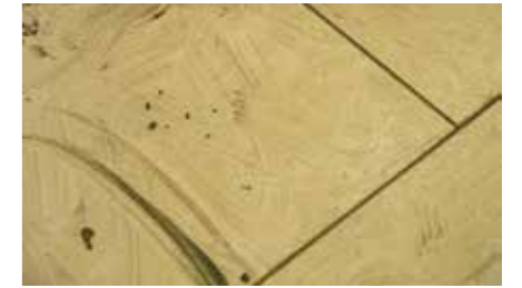
Suelo con restos cementosos / Floor with cement rest.
